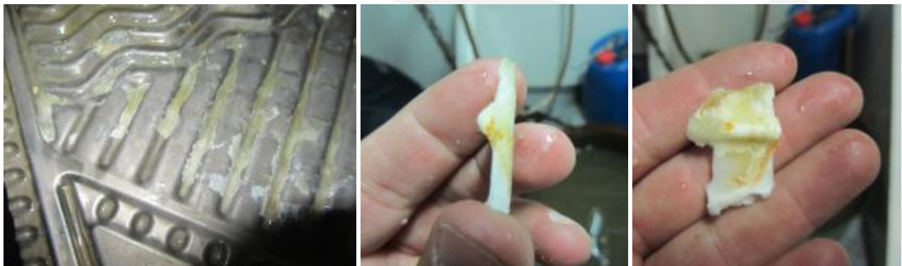
Figure 2. Lime scale precipitation on the titanium heat exchanger plates prior to the installation.
