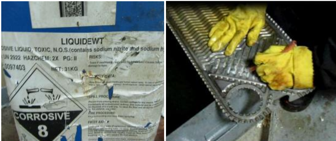
Figure 5. Left: Chemical used to soften lime scale. Right: Carving out lime scale.
