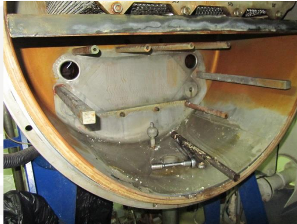
Figure 12. June 2013 - FWG chamber (where plates are mounted) treated with a HydroPath MARINE system, without any lime scale or slime.
